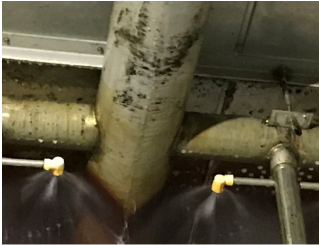
Spray Header Piping Before ProMoss™
