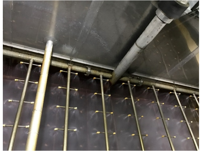
Spray Header Piping ProMoss™ Program
