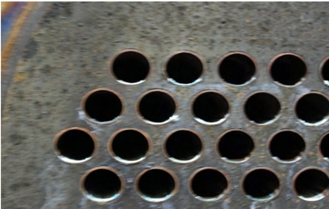
Chiller tubes from phase one test facility after two cooling seasons on ProMoss™
