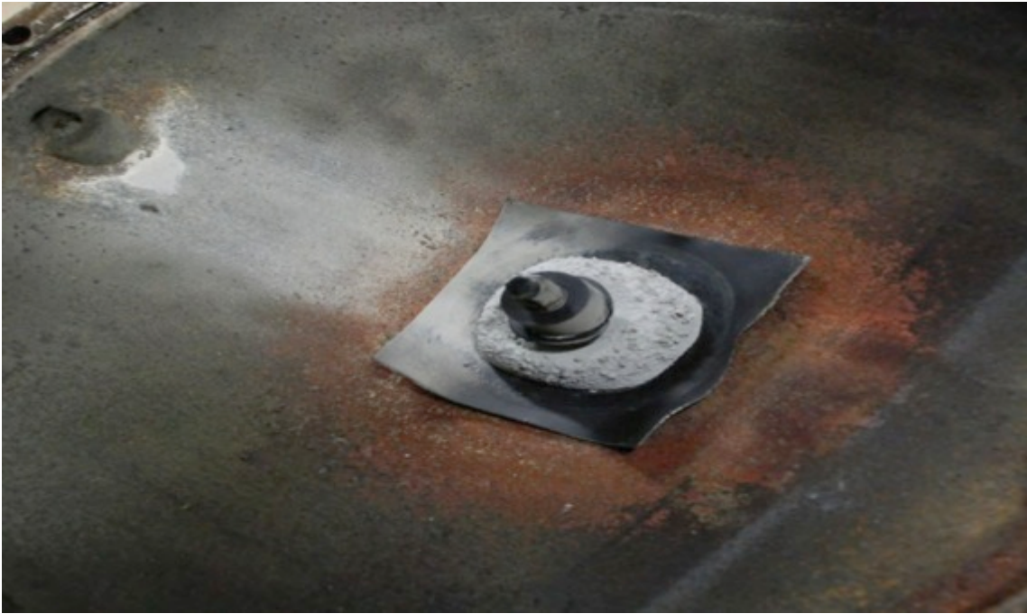
Chiller lid from phase one test facility after two cooling seasons on ProMoss™.
