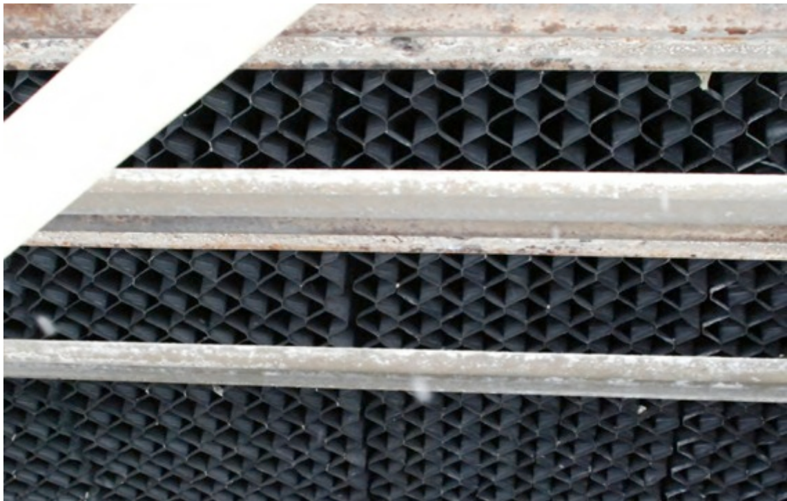
Cooling tower media from 16 year old phase one test facility after two cooling seasons on ProMoss™
